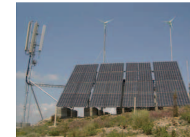
Remote Telecommunication System
