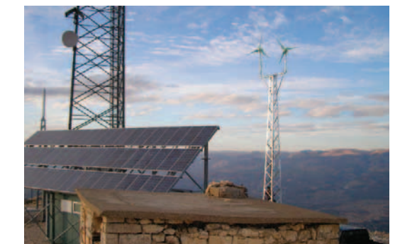
Remote hybrid wind/PV telecommunication system in Turkey
